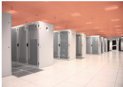
Ceiling protection at Data center
